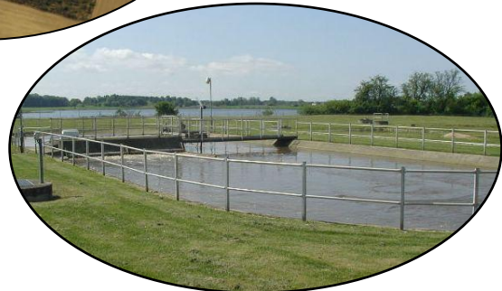
Kagerup Wastewater Treatment Plant
