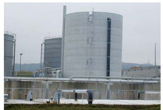
Trickling filter in industry with 16 m media depth Region Basel, Switzerland
