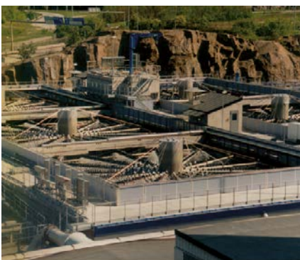
Nitrification Filters, Gothenburg, Sweden
